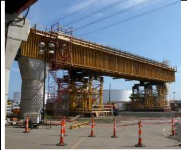
5. Form for concrete cap construction, including intermediate supports, panel forms, stairway access. (Schexnayder)
