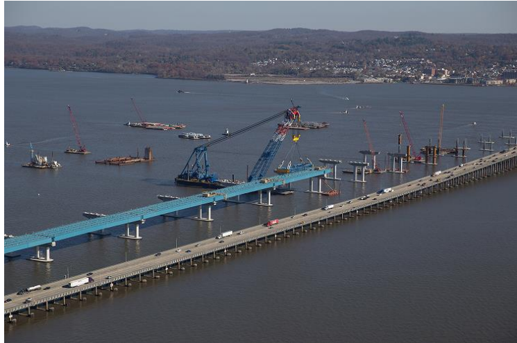
Figure 6 - Steel erection progresses with various stages of substructure seen advancing to the right and the old Tappan Zee bridge in the foreground
